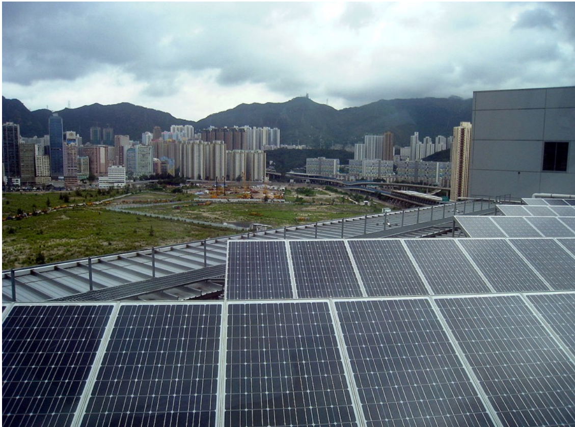
Array of solar panels on a rooftop - Hong Kong
